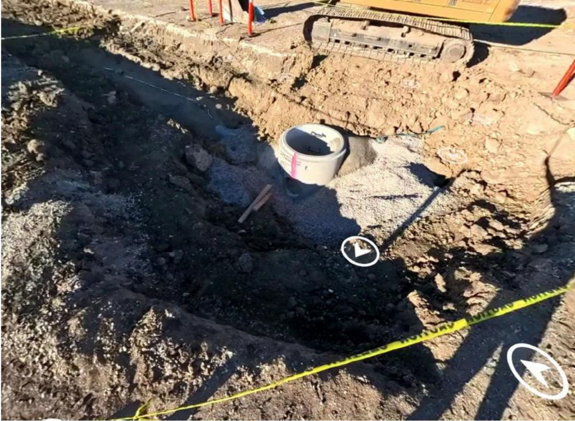
Figure 7: One of Various Storm Structures Installed
