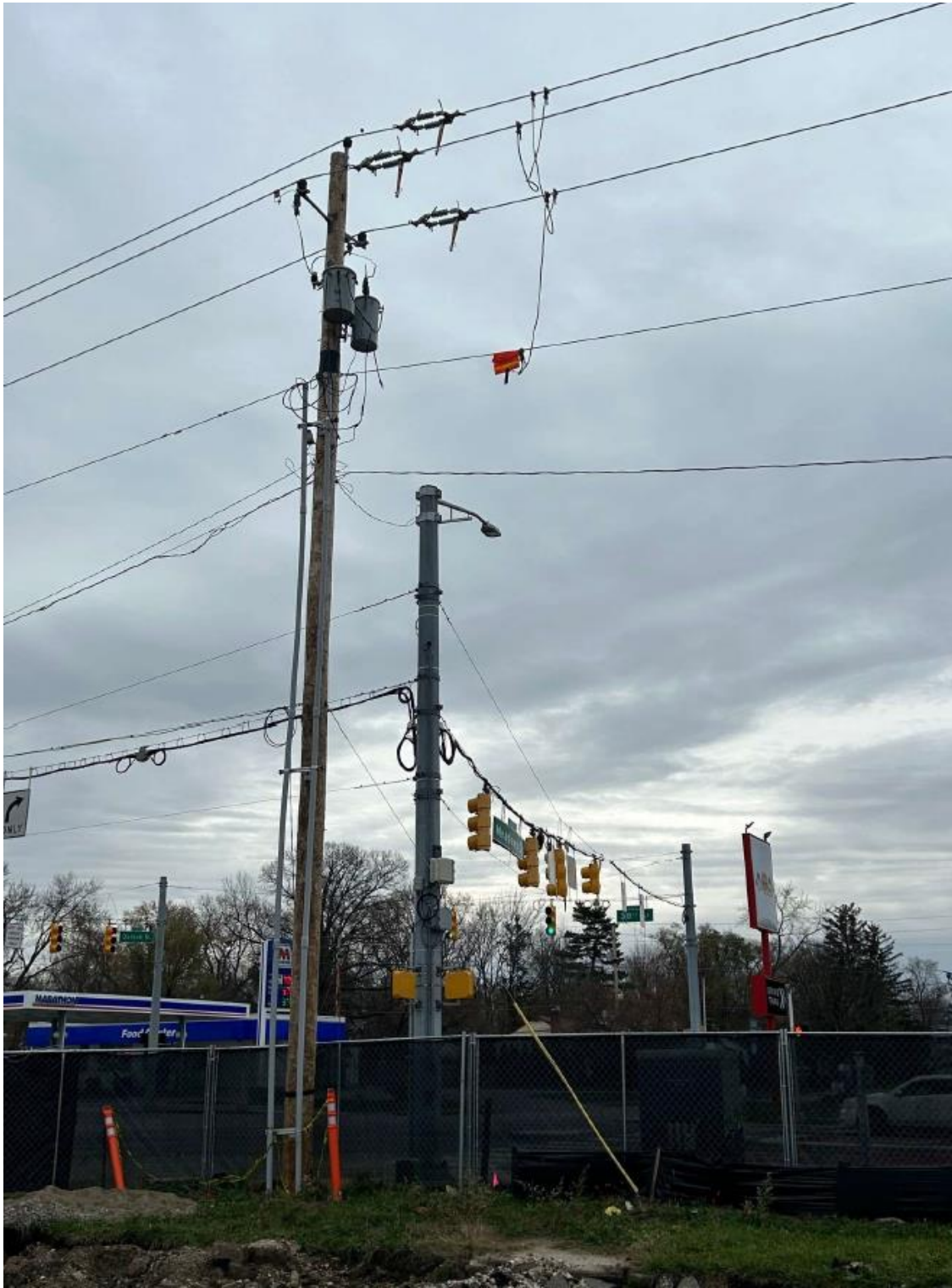
Figure 6: South Power Line Deenergized and Grounded for Safety Concerns During Building Construction
