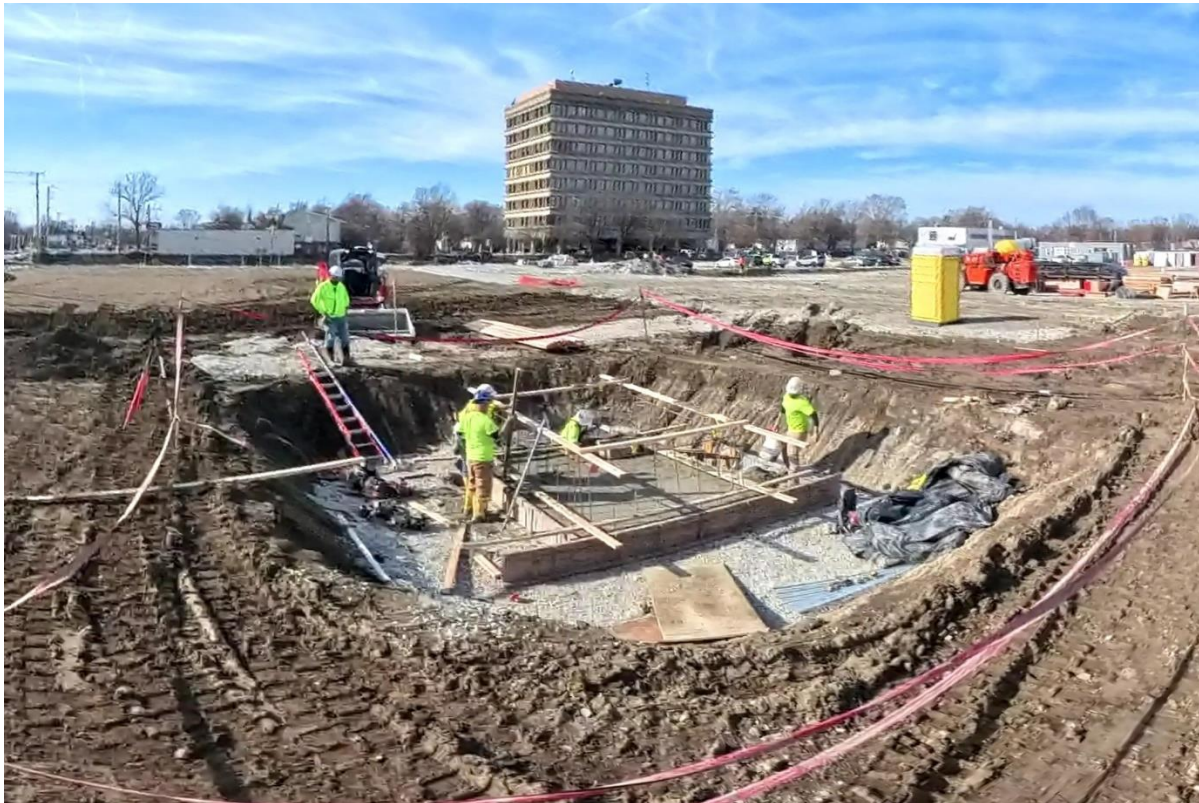
Figure 1: Setting of the Elevator Shaft, located in the central corridor of the building.
